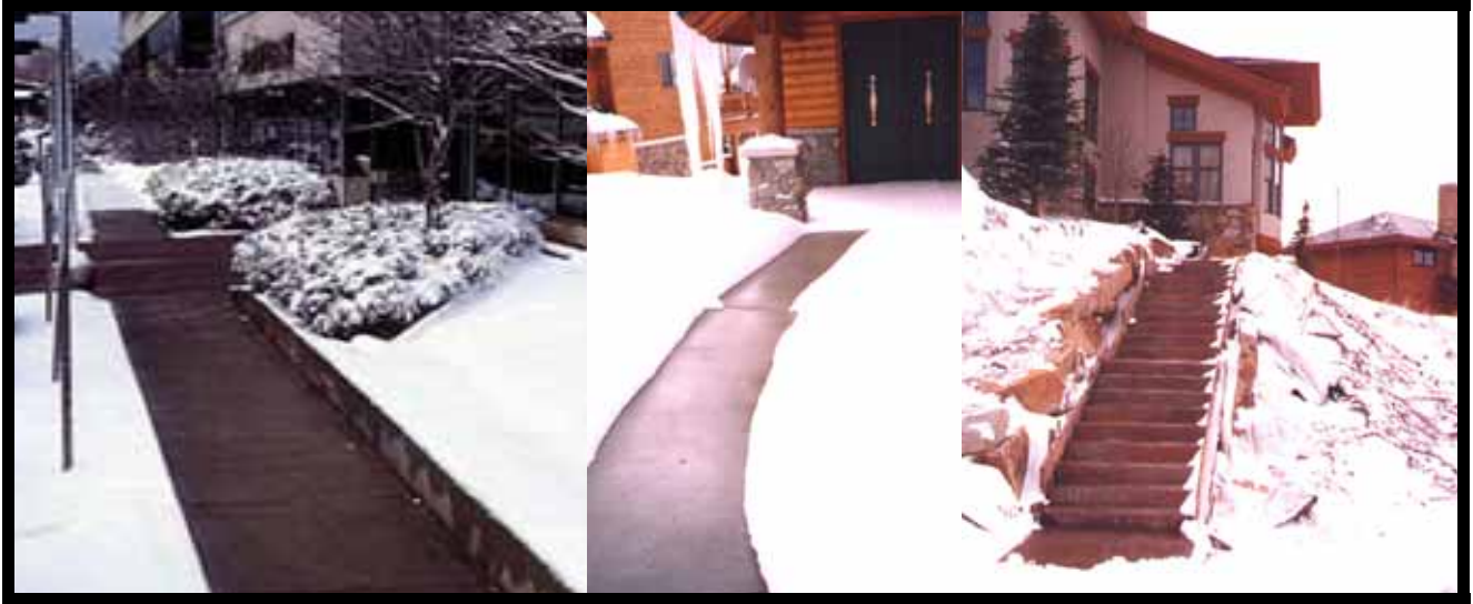
Stairs and Walkways with Tuff Cable
